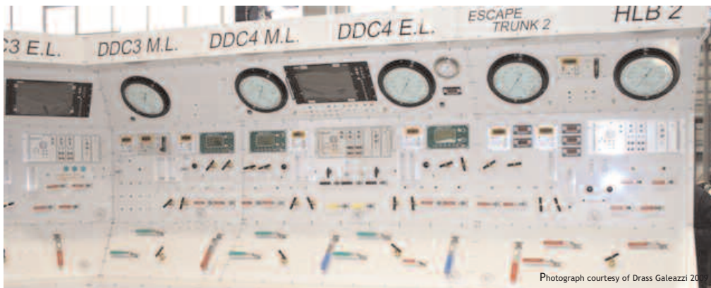
Example of a main control module mounted within a saturation dive panel.
